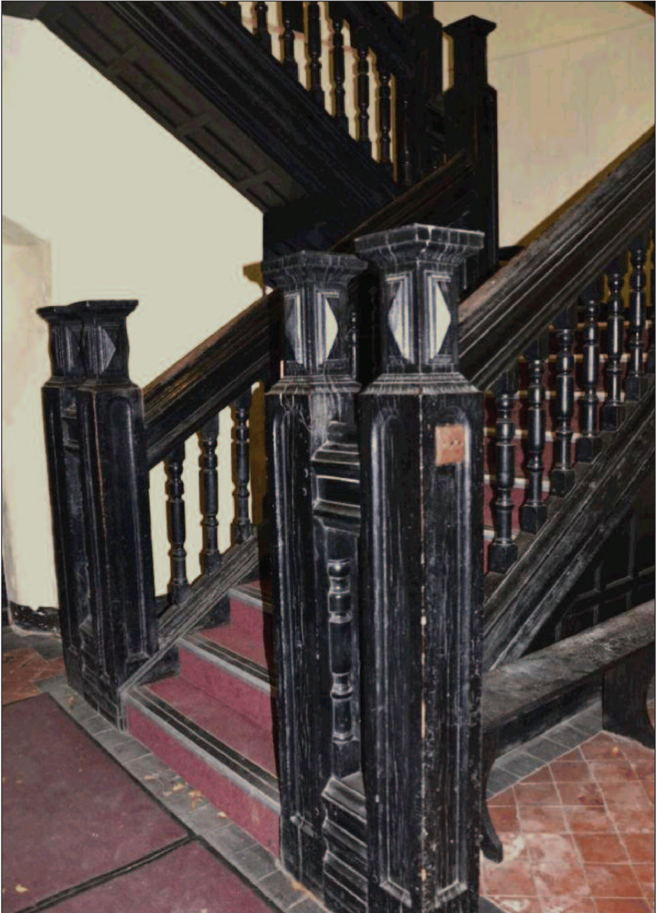
A familiar sight to all those who studied or worked at the College – the Jacobean staircase leading to A Block.
